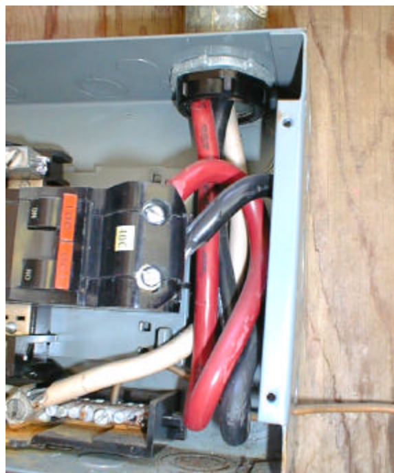
Figure 1 – Insufficient wire bending space
